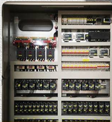
High and low power distribution cabinet
